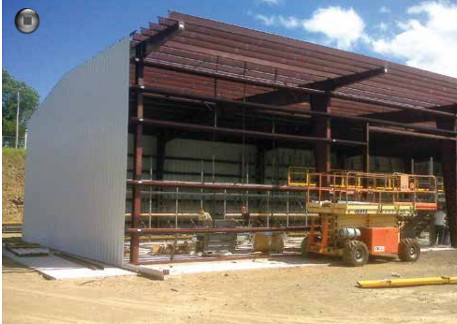
The new warehouse at LaGresley Home Building Centre has cantilever racking (L-shed) on the exterior of the building.
